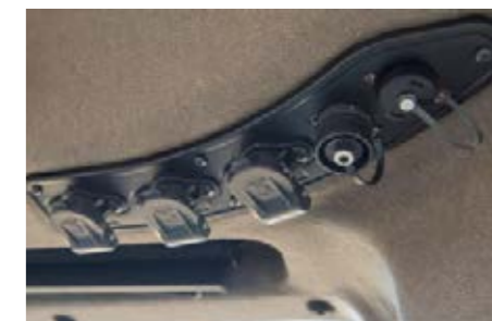
Power connections for external consumers are tidily arranged and can be easily accessed in the roof area.
